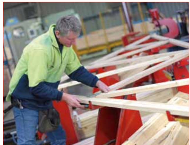
Trusses are made in precision jigs so there is uniformity of the roof planes
